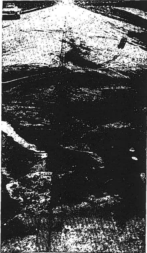
Figure 9. Both vehicles came to rest at this point. Note extensive spalling of concrete from intense heat.
