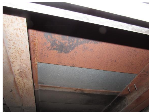
View of bus floor directly above batteries
