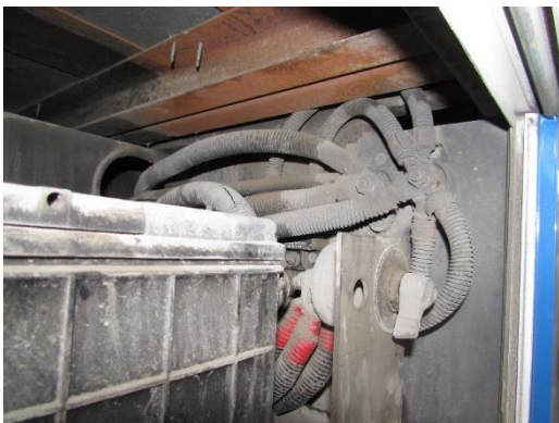
Additional view of battery cable routing
