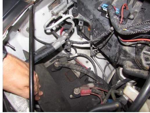
Showing battery under/adjacent HVAC
