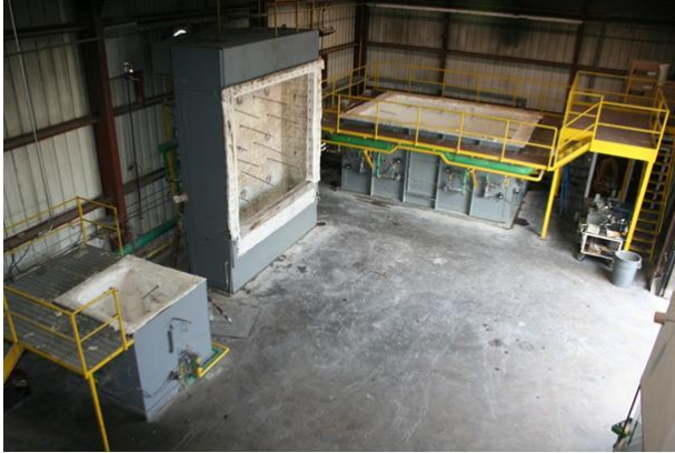
Figure 1. SwRI's fire resistance furnaces
