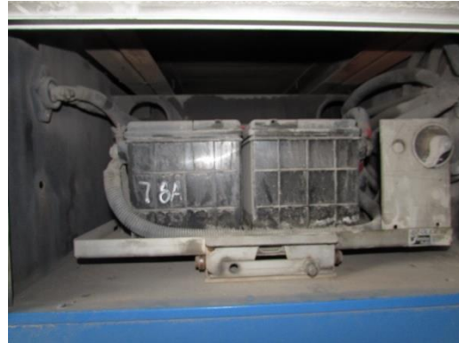
Close-up view of supplemental batteries and associated cabling
