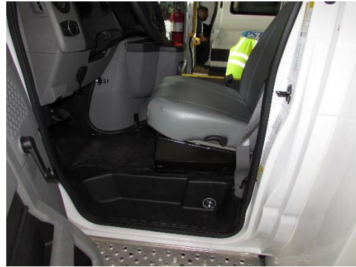
View of interior and battery disconnect switch on bottom of driver's seat
