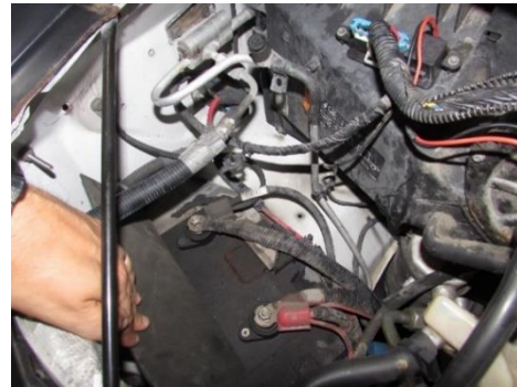
Showing battery under/adjacent HVAC
