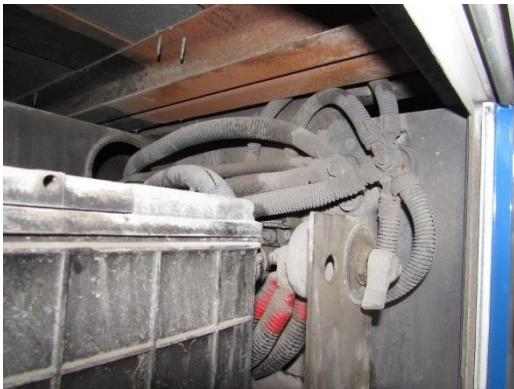
Additional view of battery cable routing
