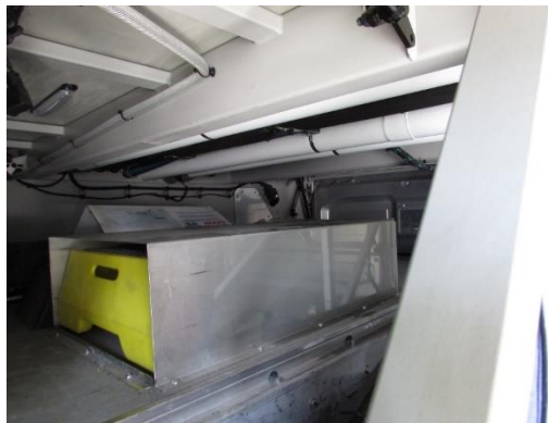
View toward rear of cable routing
