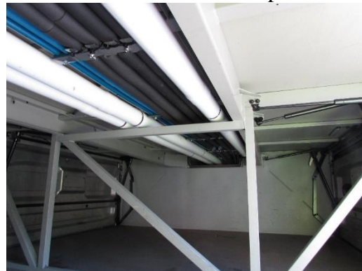
Cable routing through luggage area
