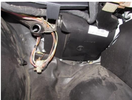
View of HVAC from interior
