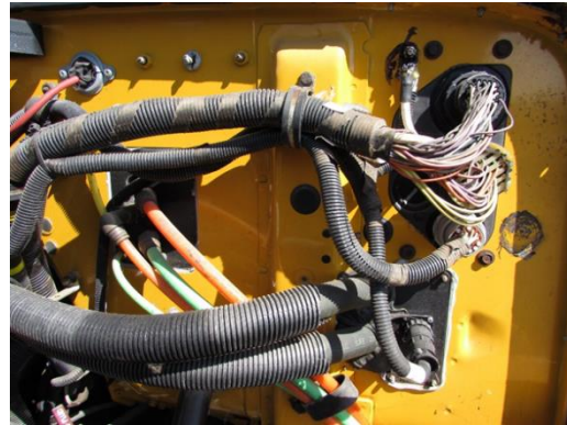
Firewall on right side
