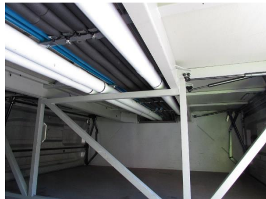
View toward front of cable routing
